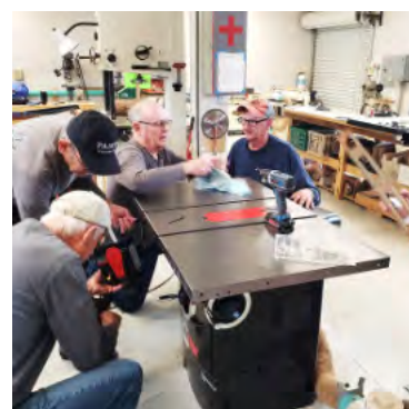
Wood Shop members Jeff Montgomery, Bill Bigelow, Terry Sander and Bob Englert install the new saw.
