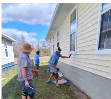
Bob Englert, Bob Slagle and Jose, the building supervisor, finish painting the foundation.
